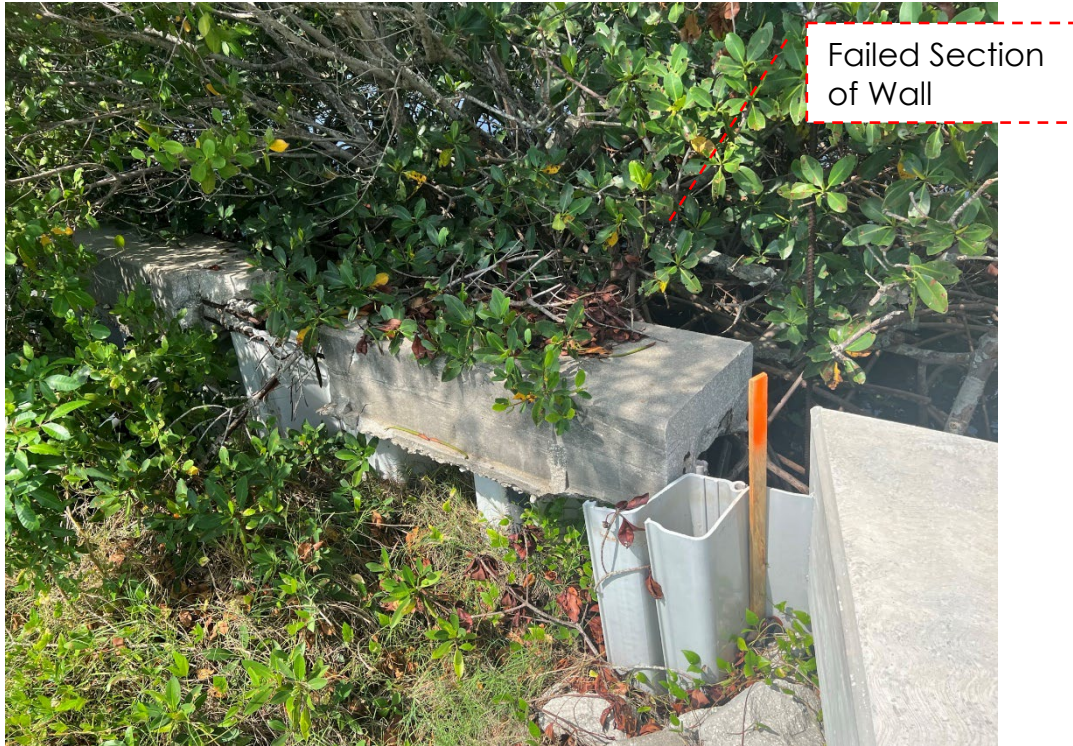
Photo #6 – Failed Section of Wall.
