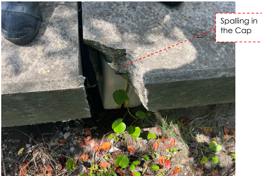
Photo #7 – Typical Spalling of Concrete Cap.
