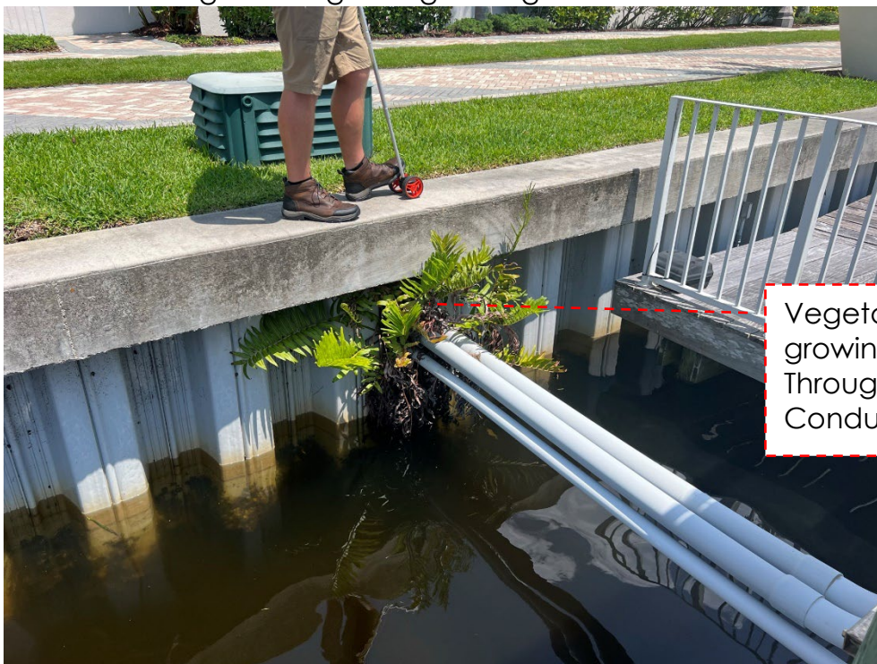
Photo #5 – Vegetation growing Through Conduit.
