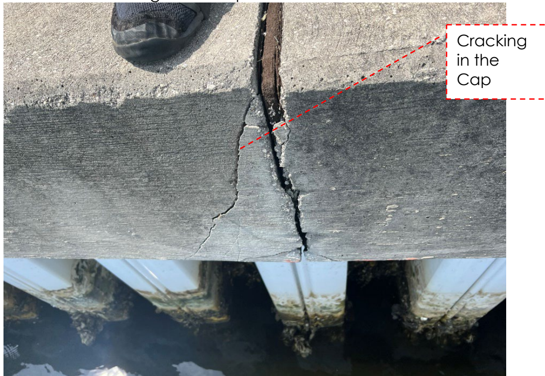
Photo #3 – Cracking in the Cap.
