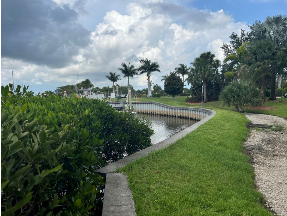
Photo #5 – Spalling in Cap. End of Section 3.
